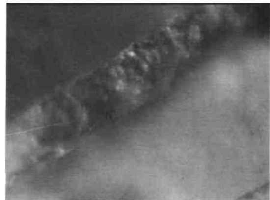
Fig.(6)' Corrosion at the borders of base of the bracket
