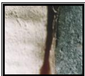
Fig. (15): Adhesive failure (X4)
